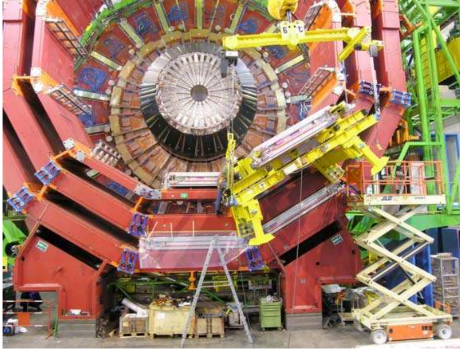
Figure 7.26: Installation of MB1 station on Wheel -2. The yellow frame is the cradle used to insert the chamber in its location inside the iron slot.
